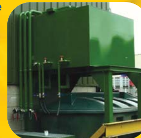
Triple compartment lube oil flask with drip tray and filler pipes on a stand to make the most of the available space.
