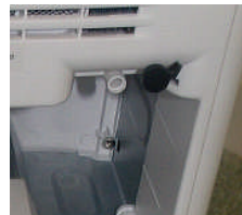
Continuous Drain Point
