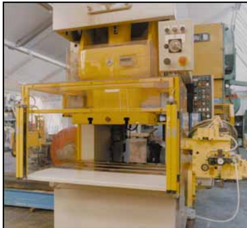
Power press fitted with a light curtain
