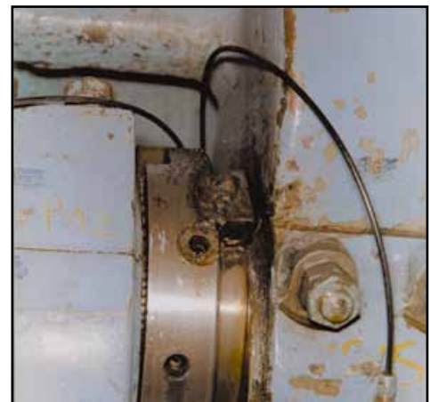
Poor standards of repair during maintenance
