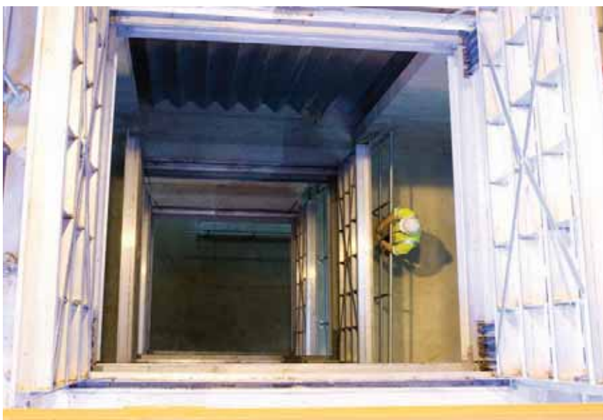
Utilities Southern Water - Folkestone - equipped with a series of 3m square JD-AL doors specially designed to withstand a 3000 kg/m 2 live load
