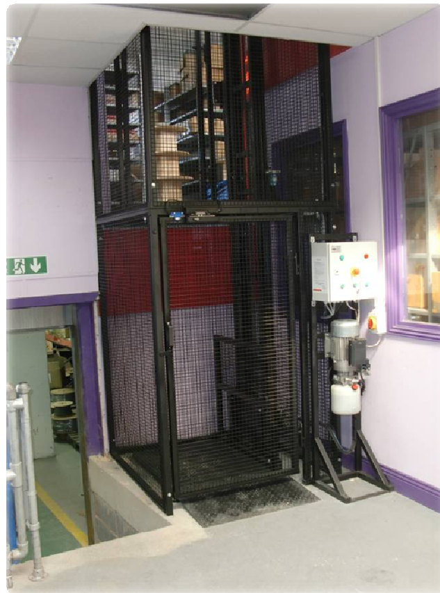
Installed at Bryant Unlimited, 70b Stafford Road, Croydon, Surrey, CR0 4NE
