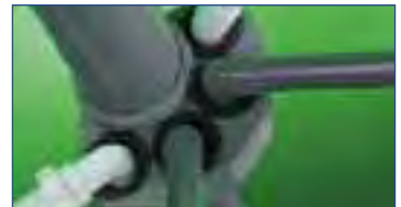
Soil & Waste Systems
