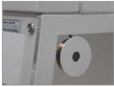
Low airflow alarm
