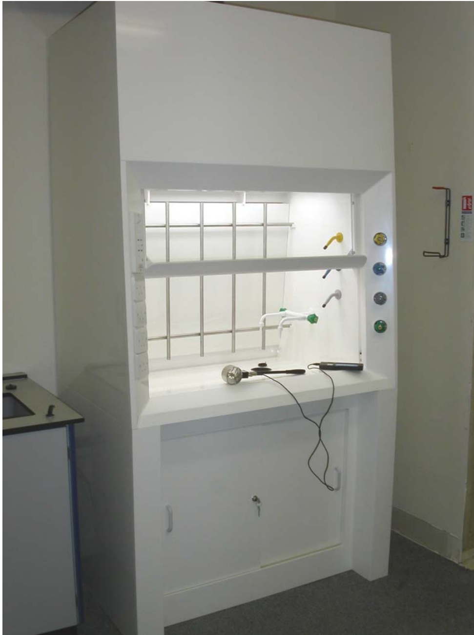
Cabinet is shown with vented undercupboard, and optional gas, water, nitrogen services and custom rear support frame
