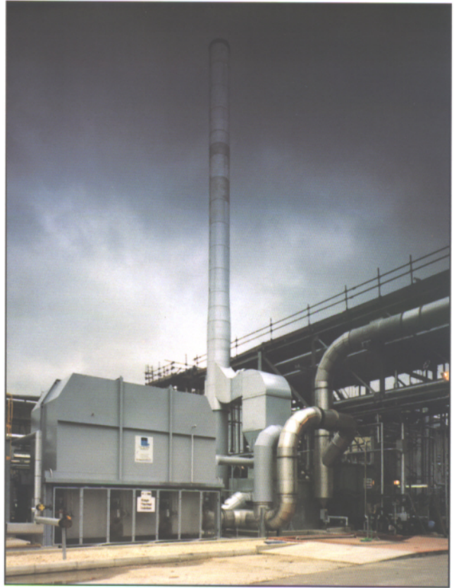
Roxitherm RTK 3-Chamber Oxidiser on Chemical Plant.
