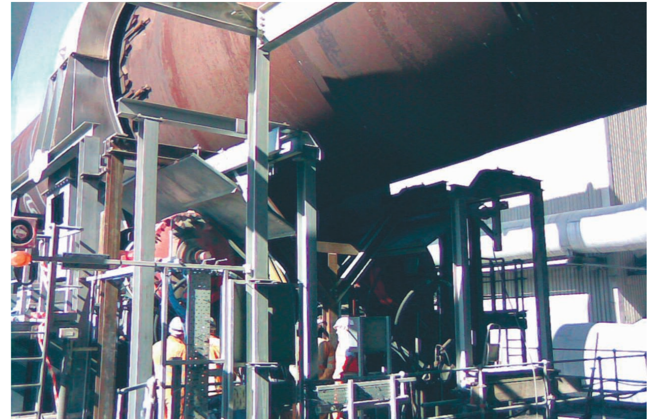
The new system was installed in February 2008 during the annual plant shut down and was successfully carried out on time.
