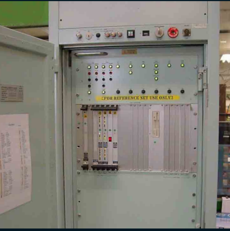
MTLS Obsolescence Upgrade
