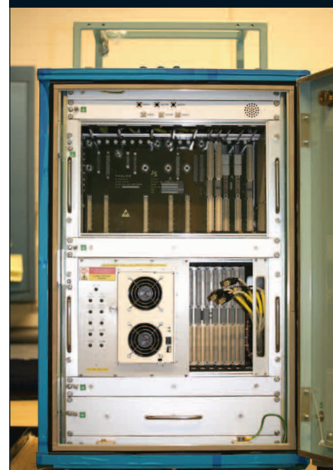
Electronic Cabinet Enclosures
