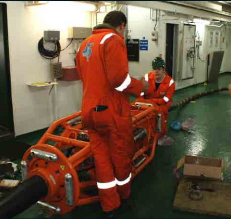
HV Power Connection
