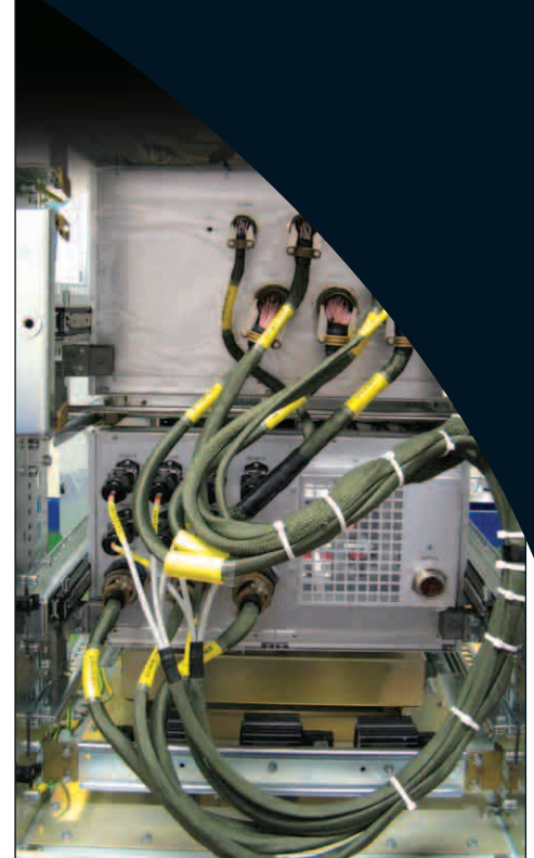
Cabinet and Console Wiring
