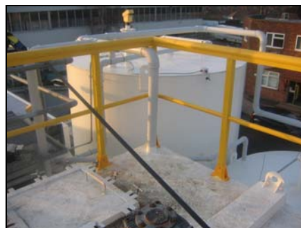
Yellow handrail system
