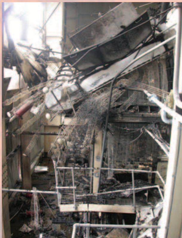
ABOVE: consequences of poor filter protection can be severe.
