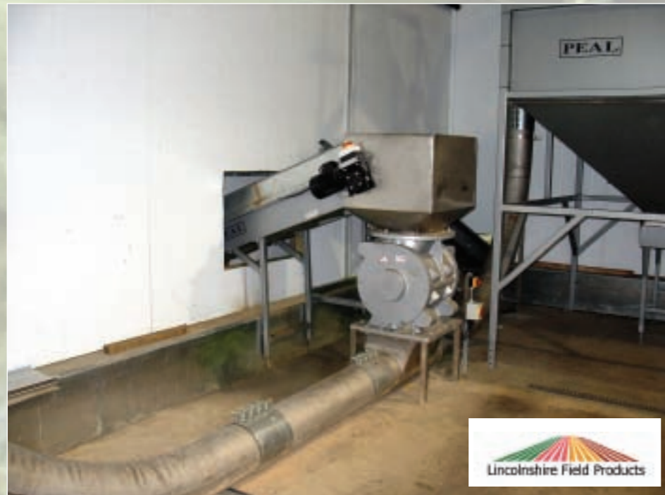
MLD 400 in use at Lincolnshire Field Products
