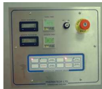
2B Controls (Flush mounted box with MBP controls)
