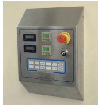
1B Controls (Surface mounted box with MBP controls)
