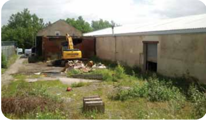
Site clearance work commences. Here an old electricity sub station is demolished.
