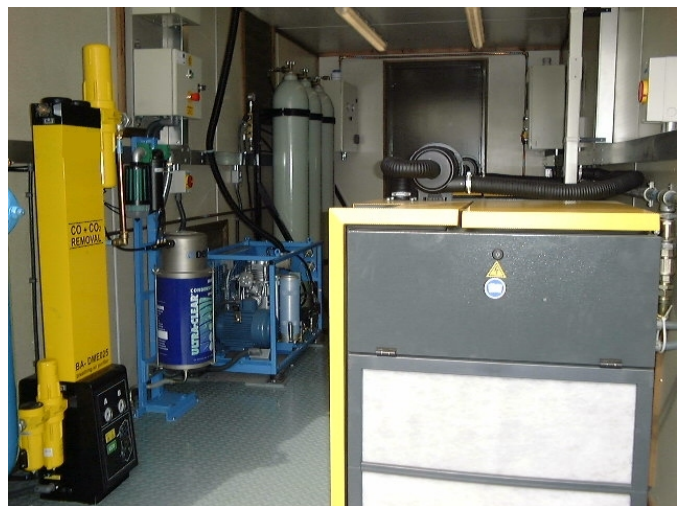
Automated breathing air system
