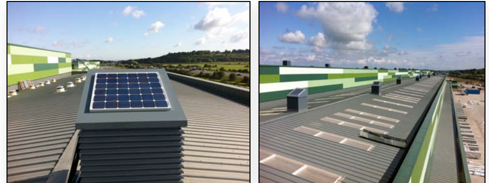
Solar Powered Roof Turrets at Morrisons Bridgwater RDC
