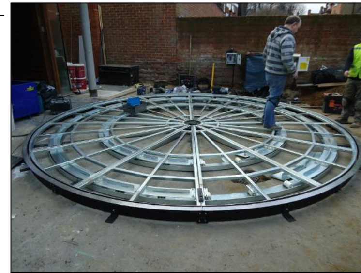
Example of Motor Housing and center bearing set in to a concrete base.
