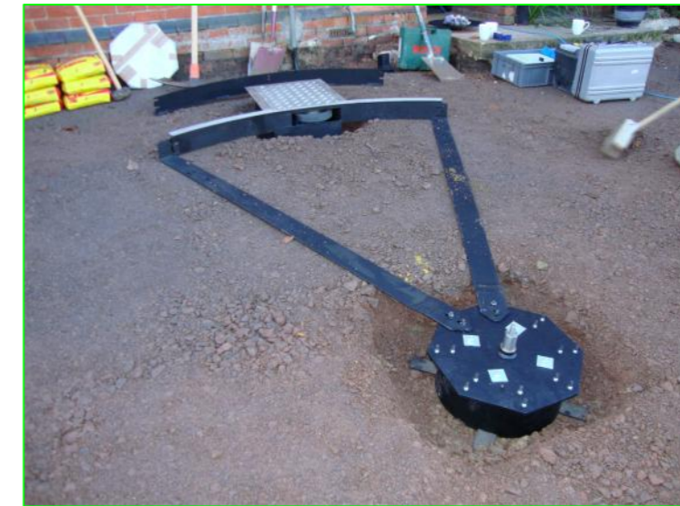
Example of Motor Housing and center bearing set in to a stone base.
