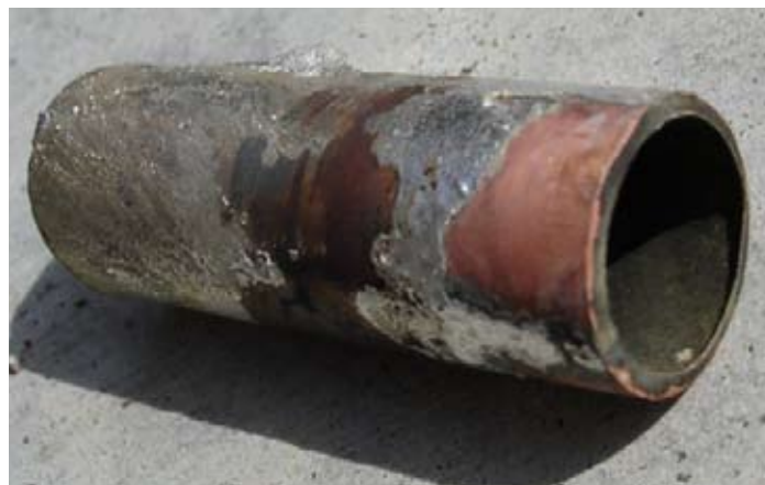
Copper pipe pin holes caused by a switch to chloramines Photo Marc Edwards, Virginia Tech.
