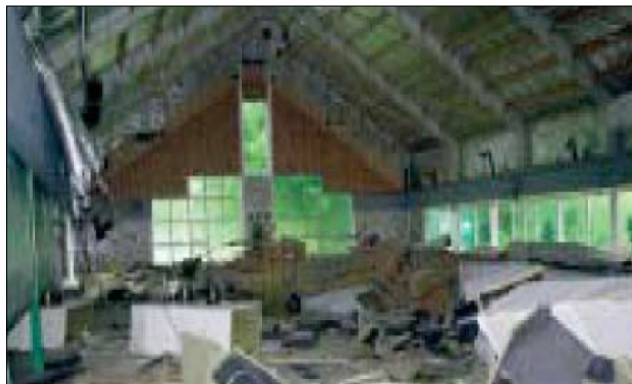
Collapsed pool ceiling in Holland caused by stress corrosion cracking.
