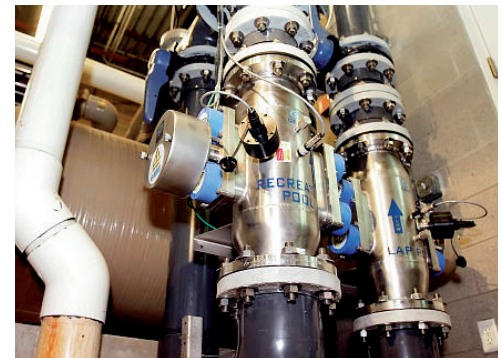
Above: ETS UV systems removing combined chlorine and disinfecting pool water in the USA.
