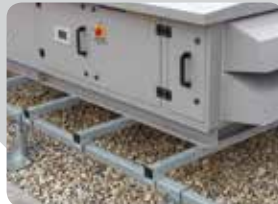
HVAC Support Frames
