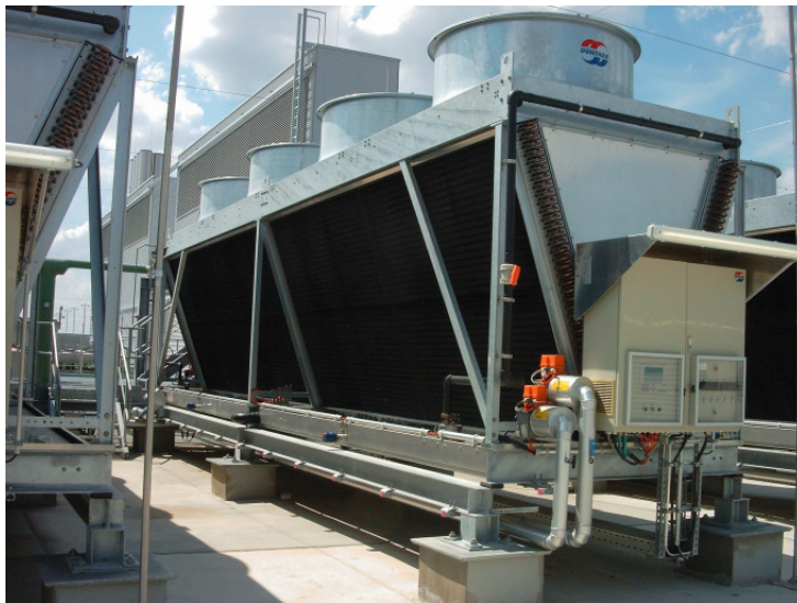
Hybrid cooler for a Data centre for SAP
