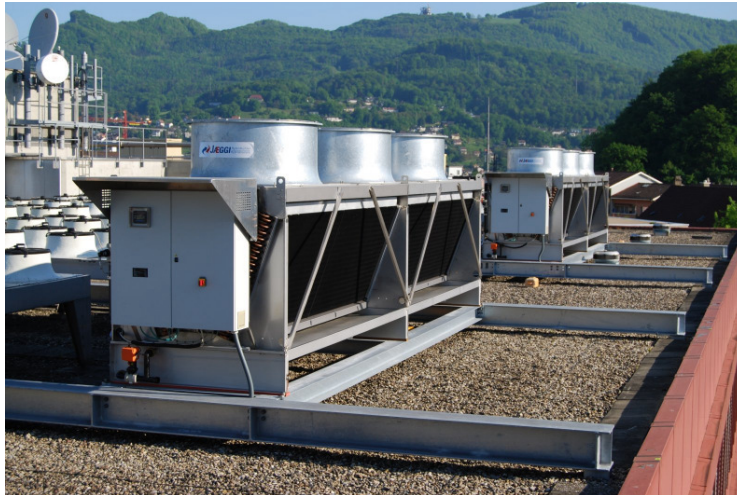
Hybrid coolers for air conditioning of computer and server rooms of a telecommunications company
