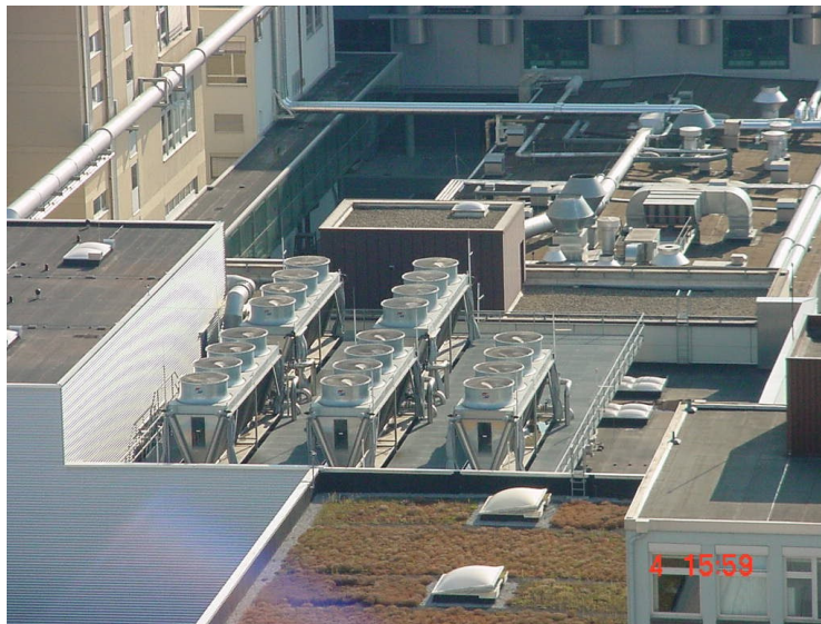
Hybrid coolers in use at an automobile manufacturer for Dynamometer cooling
