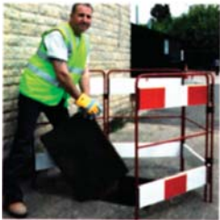
Hazard Moorgate barrier
