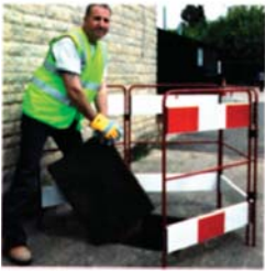
Hazard Moorgate barrier
