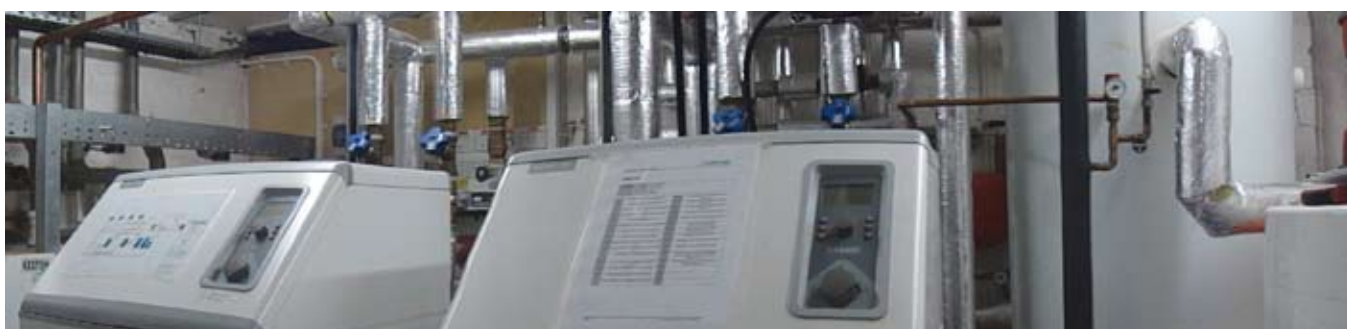
Heat pumps in the plant room
