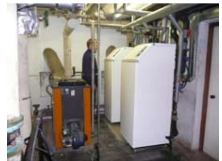
Now with one boiler for back up and two heat pumps
