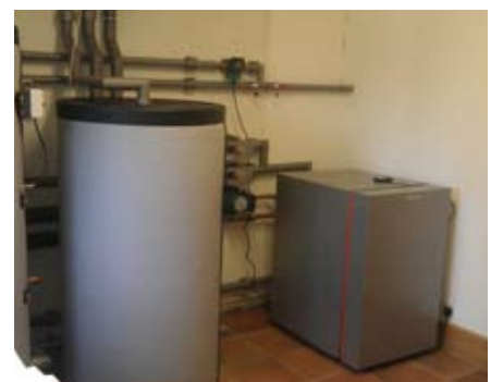
Heat pump and buffer tank in the plant room
