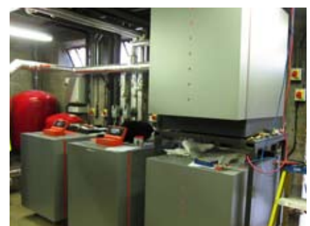
Four heat pumps installed
