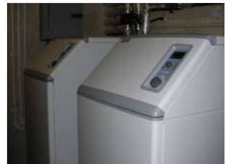
Two heat pumps in the plant room
