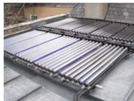
Solar thermal system on the roof
