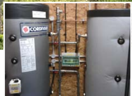
Tanks in the plant room awaiting insulation
