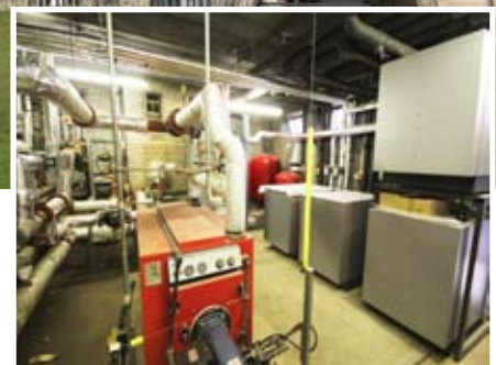
Plant room showing heat pumps and back up boiler
