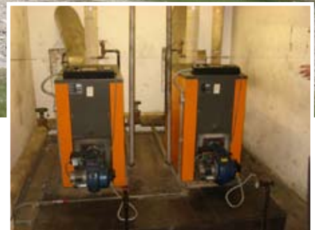
Original plant room showing two boilers
