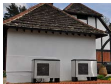
The two heat pumps
