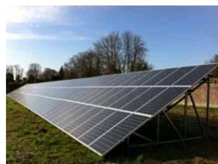
Ground mounted solar photovoltaic system
