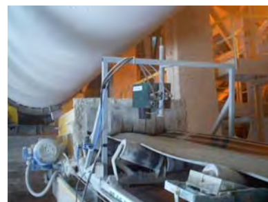
Exit of the drum drier.
