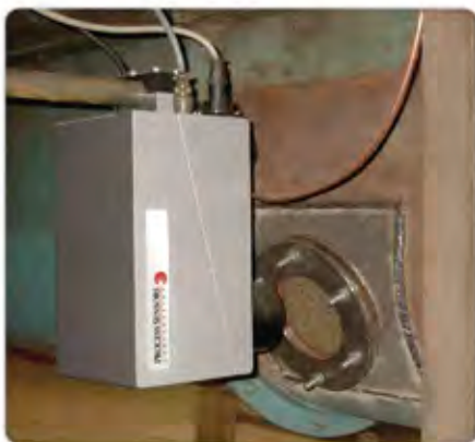
Moisture through sight glass
