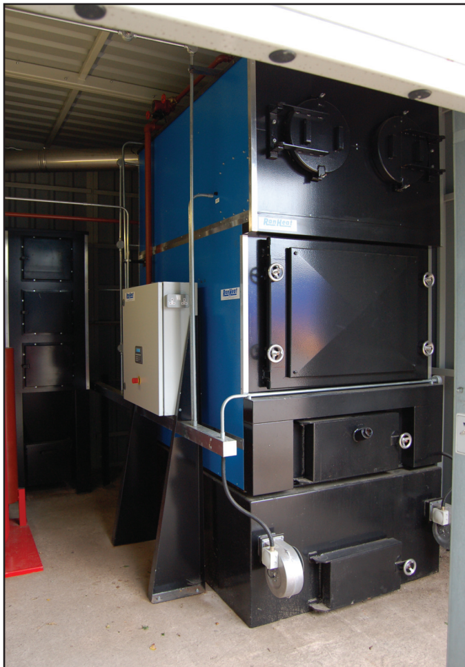
The increase in the use of economisers has been driven by government legislation and grants.
