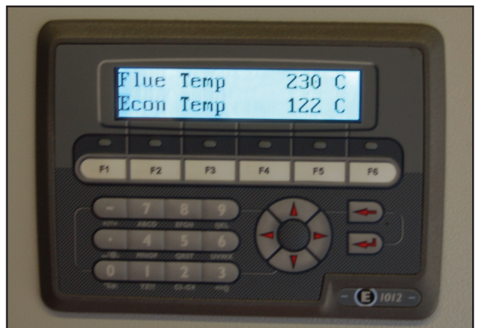
The economiser typically reduces the flue temperature by over 100 °C.
