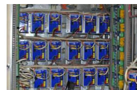
One of the Omniflex panel internals showing TR modules in the confined space
