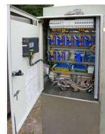
Omniflex CP system at Cardinia Creek
