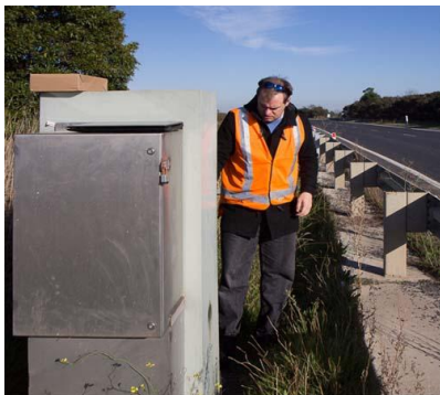
Luke Thompson, Technical Manager for Infracorr during system commissioning.
