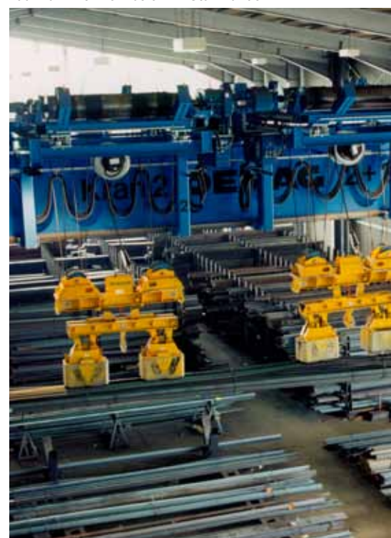
Overhead crane with two trolleys in a steel trading company
