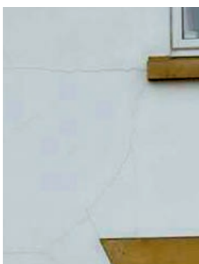
Cracks - Painted Surface
