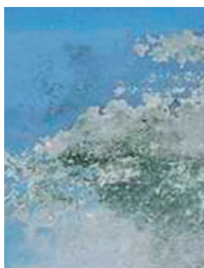
Efflorescence - Painted Surface
