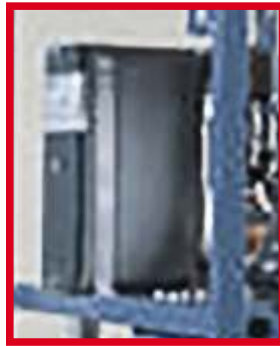
The M10 in Swedewater's system.
