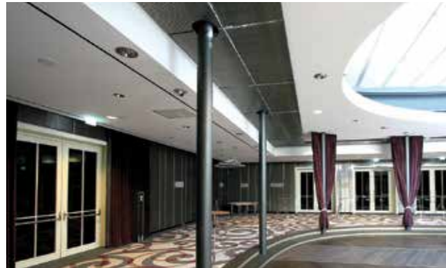
Chilled ceiling, Hotel Steigenberger Drei Mohren, Augsburg, Germany. Architect: Alpstein. Mesh: Atlantic (5)
