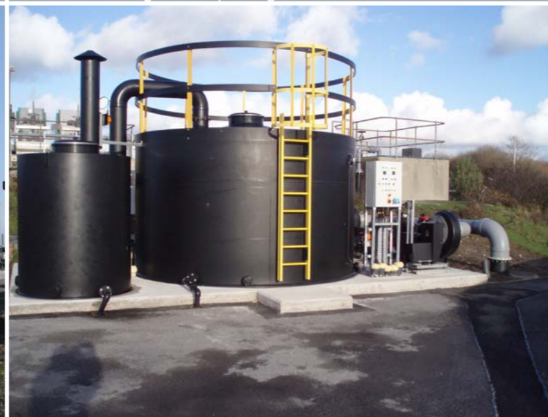
▼ Biotrickling filter with polishing carbon for Welsh Water
