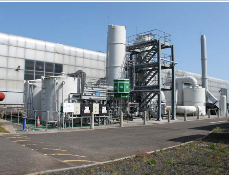
▼ Two stage wet chemical scrubber with carbon polishing filter at Kirkcaldy
