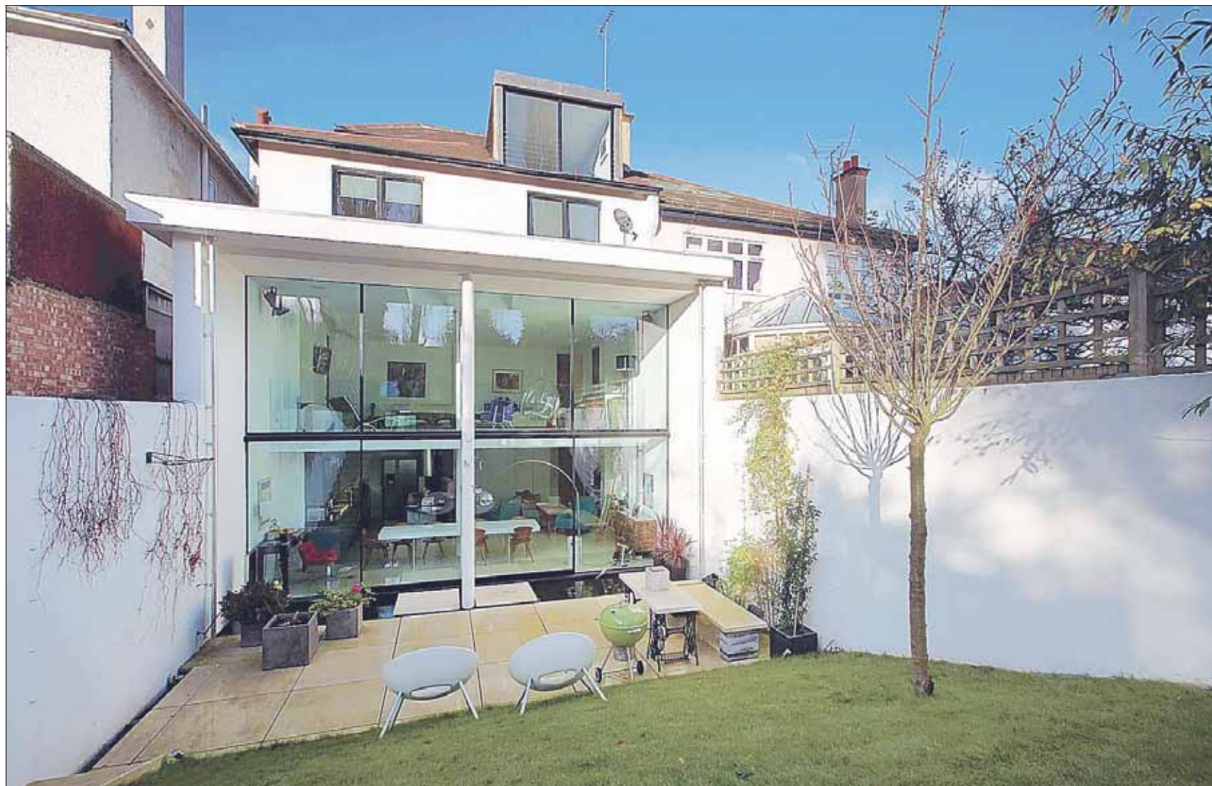
The level of the garden was lowered and the back half of the house was demolished and replaced with double-height glass, changes that allowed the original basement space to be transformed
