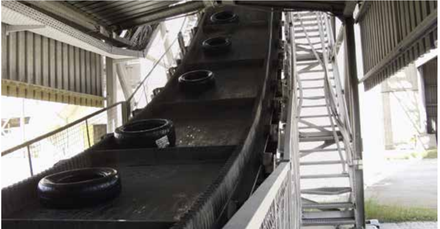
A flat belt conveyor with corrugated side walls lifts whole tires from the ground level to the point of feeding at the preheater.
