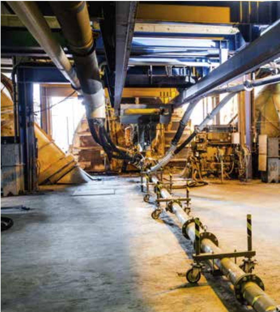
Pneumatic conveying line to the main burner
