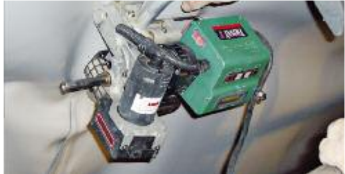
TWINNY T, with convenient cross-handle, at work overhead welding in a tunnel.
