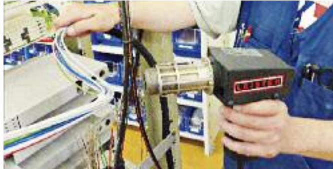
The GHIBLI forming electrical cables.
