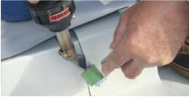
HOT JET S with angled nozzle welding a T-joint on the roof.
