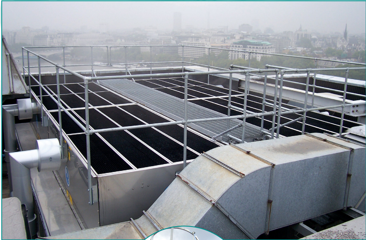
Casing perimeter handrail system
