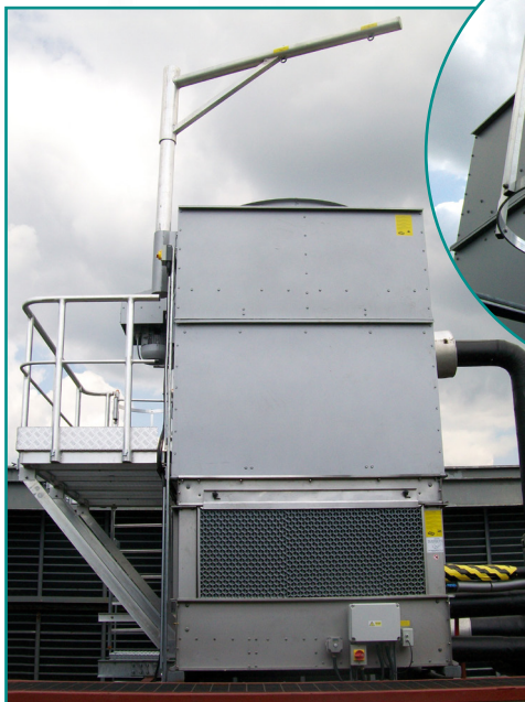
Platform complete with kickboards and motor/fan davit
