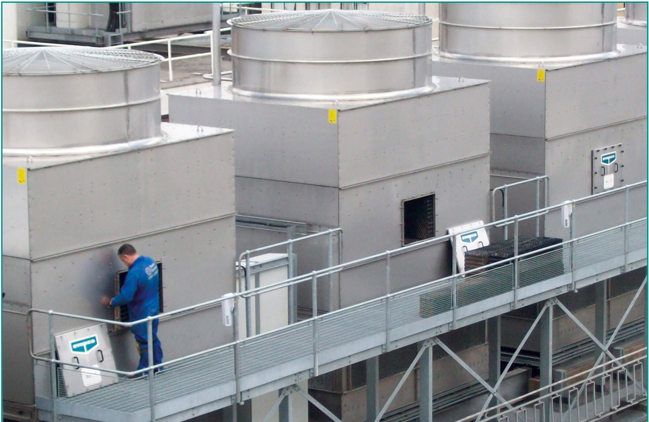
Custom design platform to enable inspection and periodic removal of fill pack
