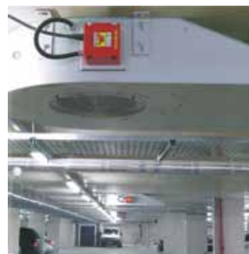
High velocity extraction fans installed in an underground car park
