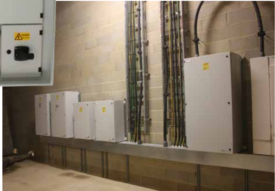
Combination ATS units with external door closed
