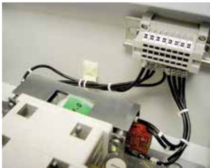
Interior view showing flag indicator and the auxiliary blocks wired down to terminals.
