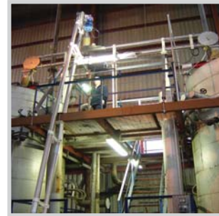
Inclined and horizontal AMCs feeding additives to either of 2 tanks.
