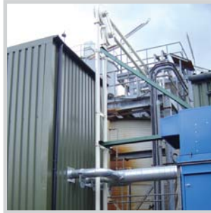
Round the corner AMC feeding chemicals to a mixing vessel.
