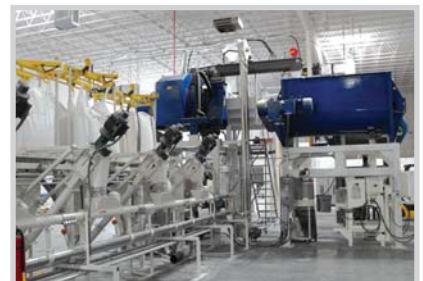
An AMC with multiple inlets delivering cement, sand, ash and recycled glass to a second unit that lifts them up into a mixer.
