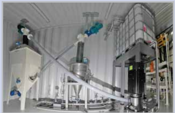
Water treatment system inside an ISO container.
