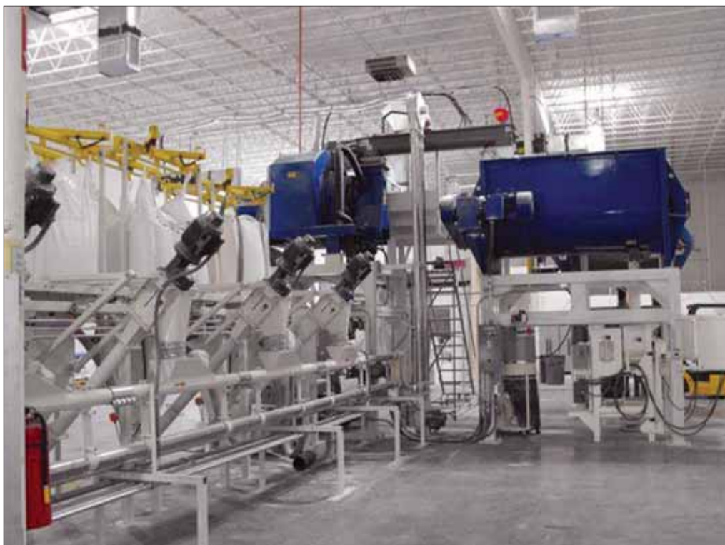
An installation in the USA which includes Spiroflow bulk bag dischargers, flexible screw conveyors and aero-mechanical conveyors.
