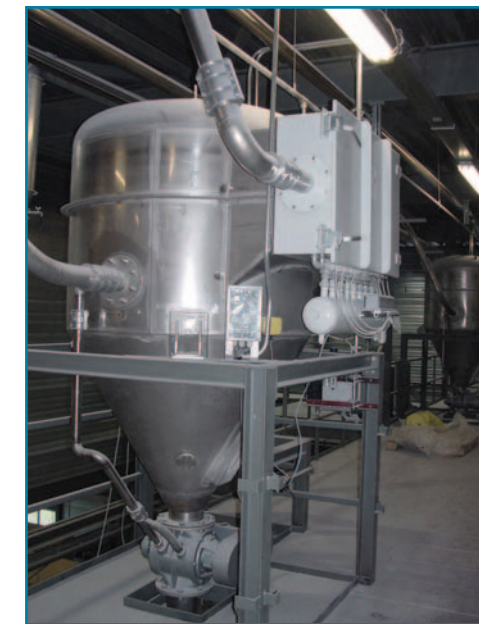
Pneumatic Conveying System
