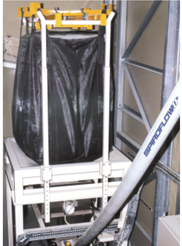
A low loading Type 5 discharger is used due to restricted headroom.
