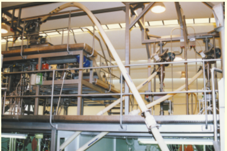
ABOVE: Flexible screw conveyors at Farley Health Products.
