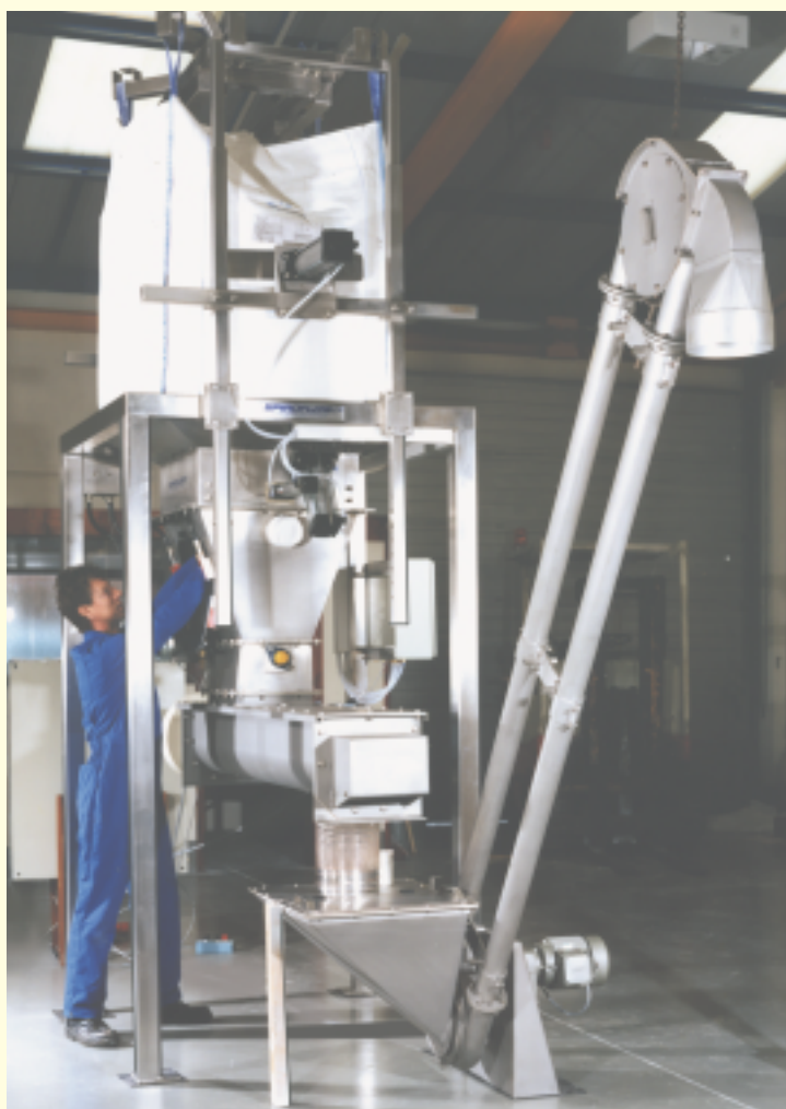
ABOVE: Bulk bag discharge system incorporating an aero-mechanical conveyor for the handling of titanium oxide.
