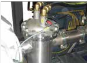
Heat exchanger to cool down the hot gas
